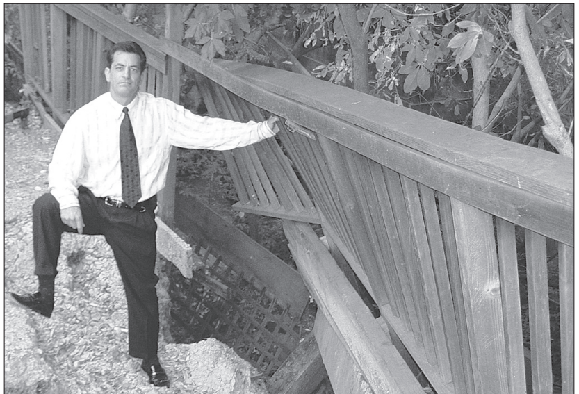
Real estate attorney Jeffrey Lerman in front of a collapsed retaining wall in Fairfax.
